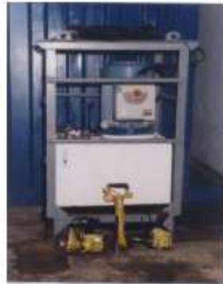
Hydraulic Power pack
