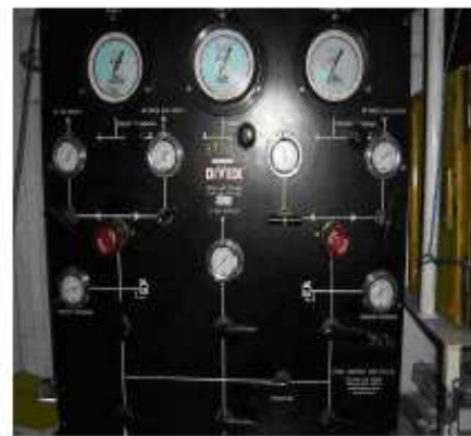
Diving control panel in control container
